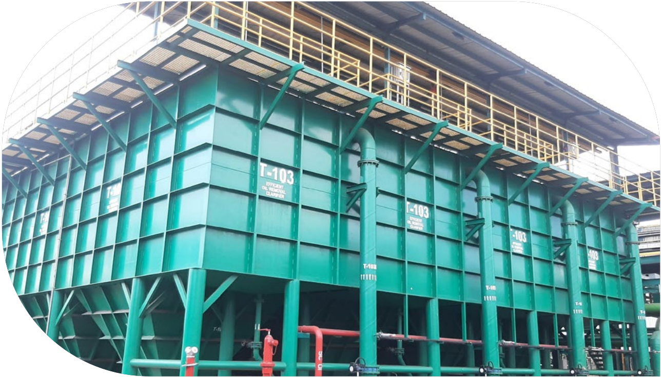
Instalasi Pengolahan Air | Water Treatment Plant
