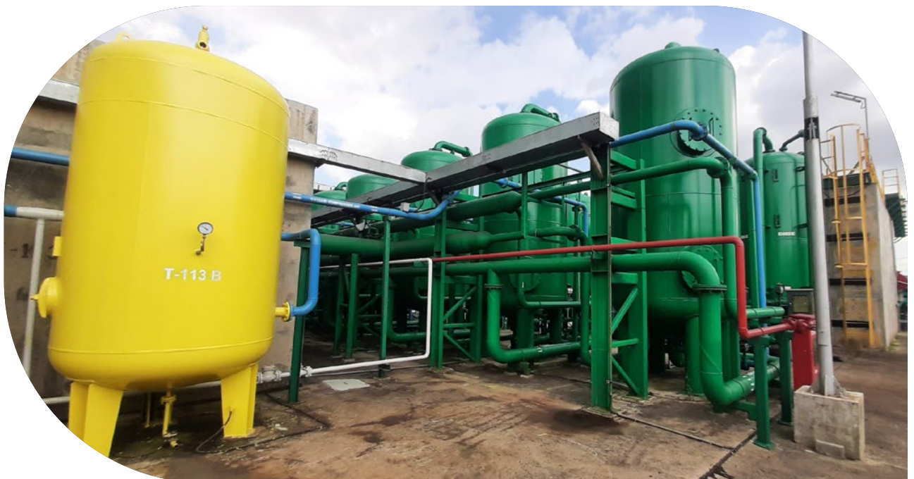
Instalasi Pengolahan Air | Water Treatment Plant
